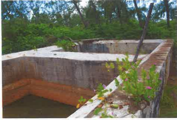
One of the two large water storage tanks, used by the inhabitants of the first Village
