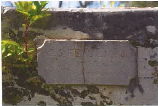
Plaque with the date of completion of the second water tank. 25 th Feb 1910.
