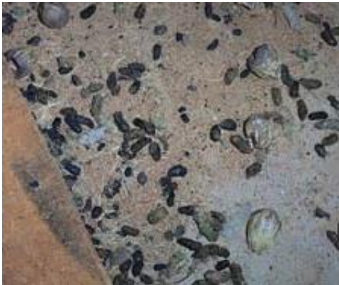
Droppings of rodent.
